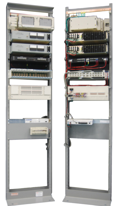
Utility Alarm Collection, Aggregation and Transport Rack
