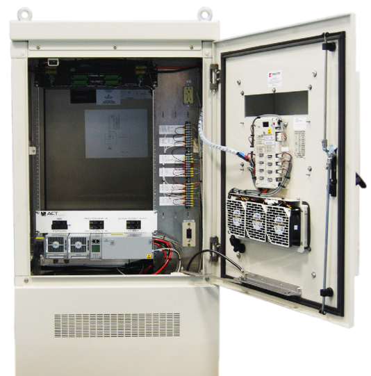
Mobile Backhaul Base Cabinet
